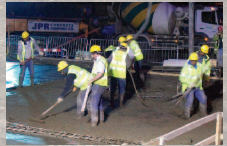
Concrete is poured into the foundations to create a rock-solid raft on which the car park will stand.
